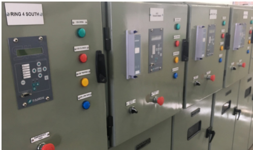
SIL-A relays installed in Azadi Football Stadium's electrical substation.
